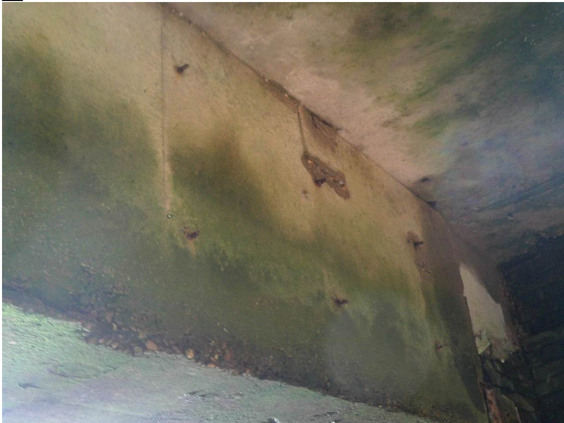
06. UNDERCROFT – SIDE OF RC BEAM WITH EXPOSED TIE BARS
