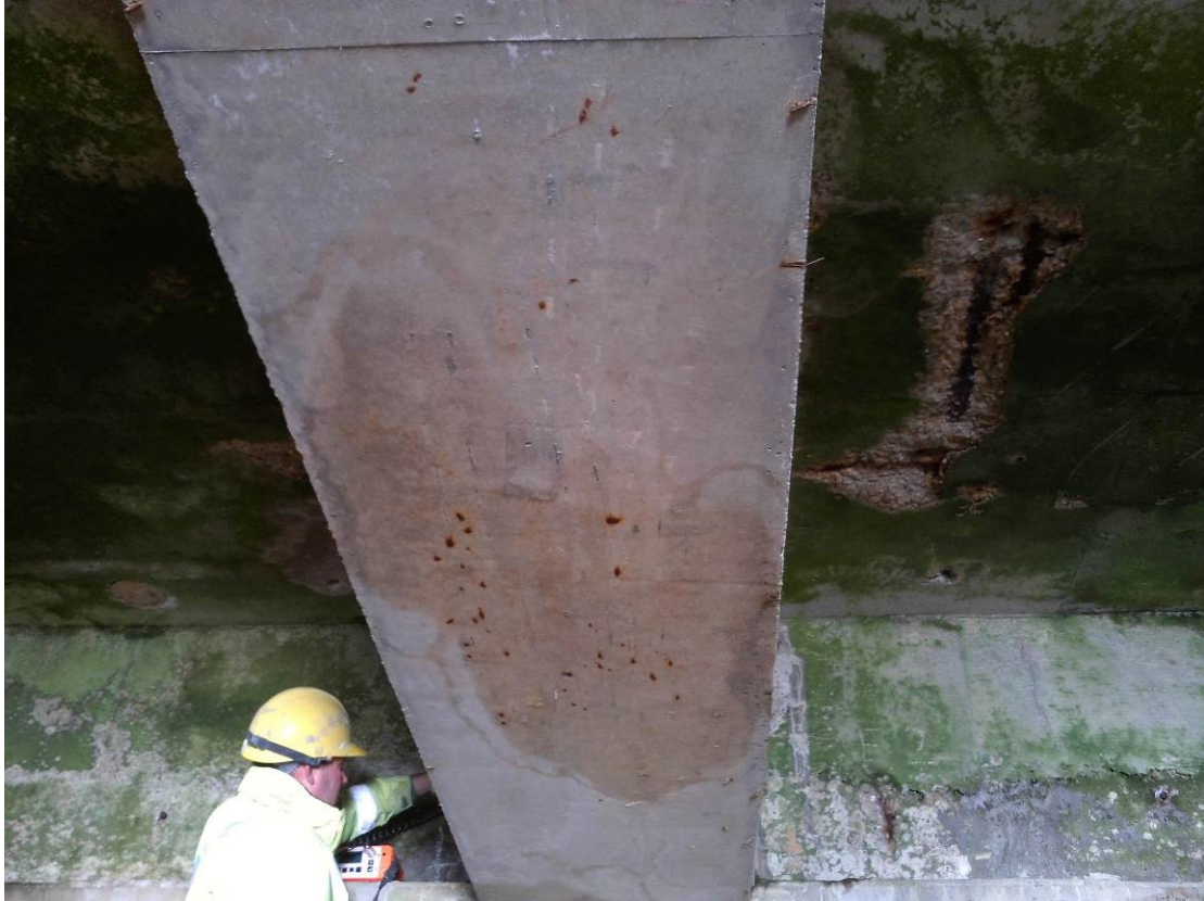
03. UNDERCROFT – SOFFIT OF RC BEAM WITH EXPOSED TIE WIRES
