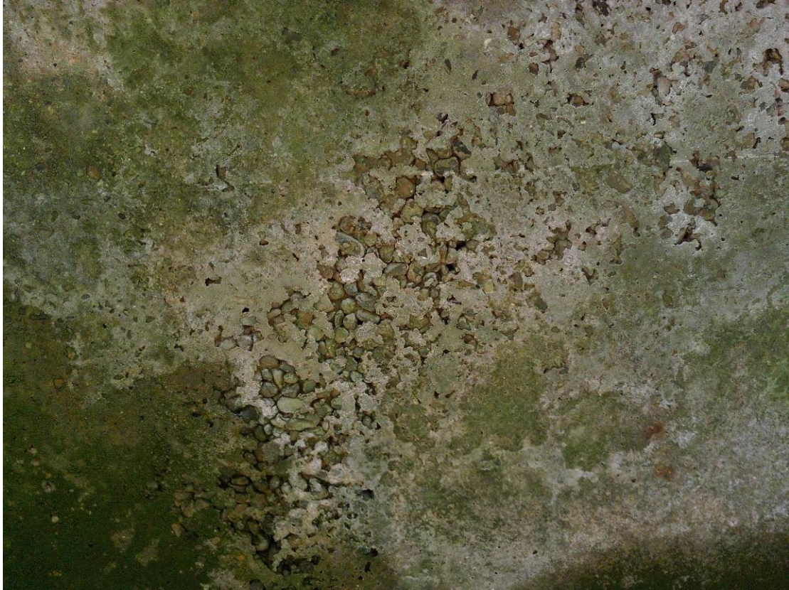
05. UNDERCROFT – SOFFIT SLAB WITH EVIDENCE OF POOR COMPACTION
