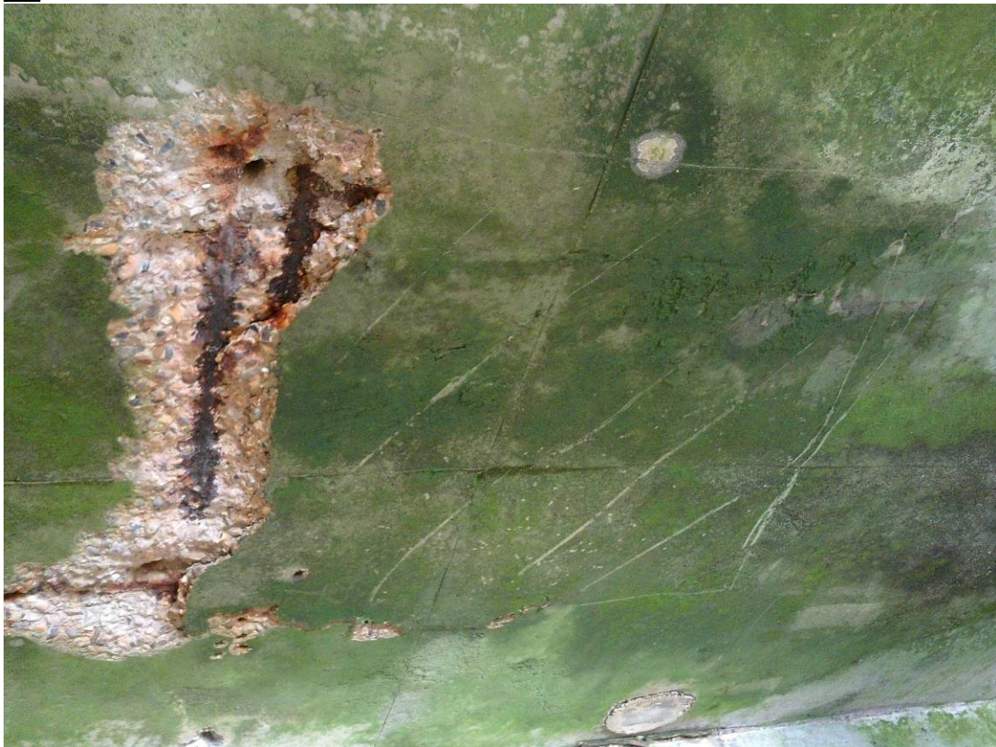
04. UNDERCROFT – SOFFIT SLAB WITH SPALLED & DELAMINATED CONCRETE
