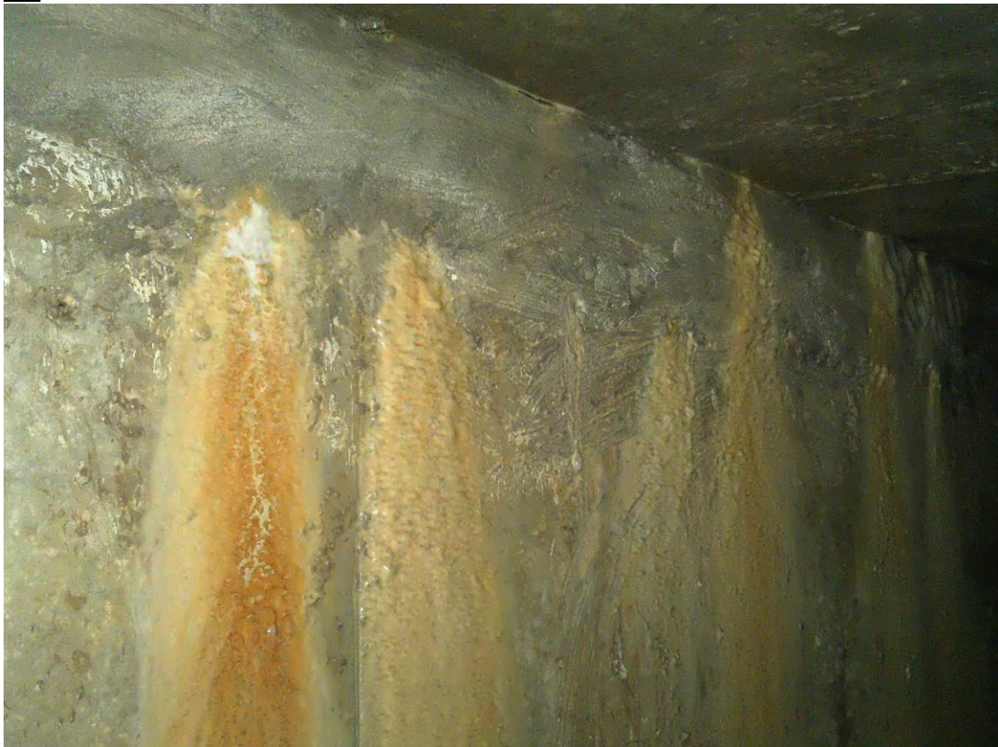
08. UNDERCROFT – LECHATE DEPOSITS ON SIDE OF RC BEAM
