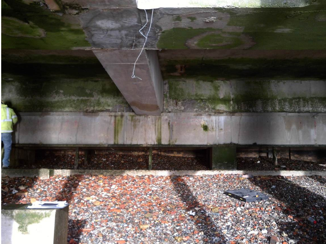
07. UNDERCROFT – SIDE OF RC BEAM SHOWING CRACKS & LECHATE DEPOSITS
